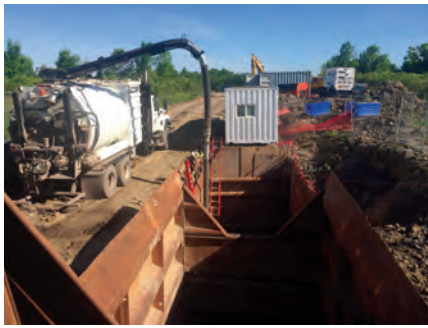
A VACUUM TRUCK WAS USED FOR SPOIL REMOVAL, WITH ALL ROCK CHIPS BEING REMOVED THROUGH A VACUUM TUBE.
